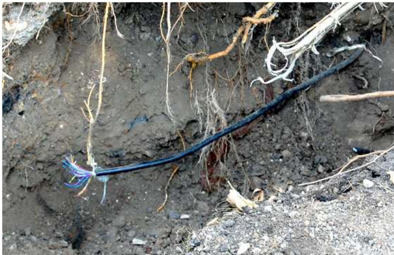
Cut cable (electrical open)
